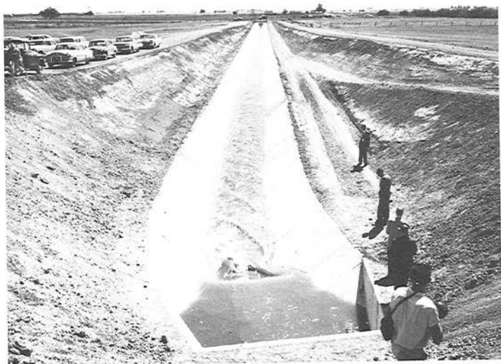
First Water Release from Putah South Canal into S.I.D.'s Vaughn Canal in 1959
